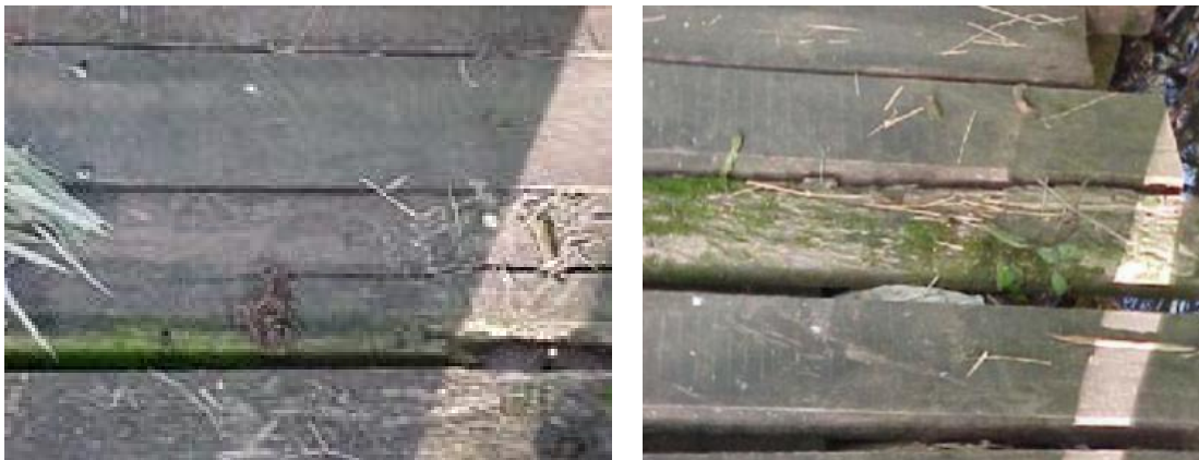
Fig. 2. Deterioration and shallow deck decay [5]
