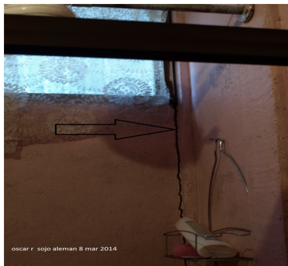
Figure 6. Cracks in the walls of a house in Barrio Fátima
